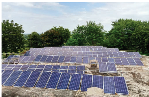
Solarization of Water Treatment Plant (WTP) in Amalner Nagar Palika (ANP)
