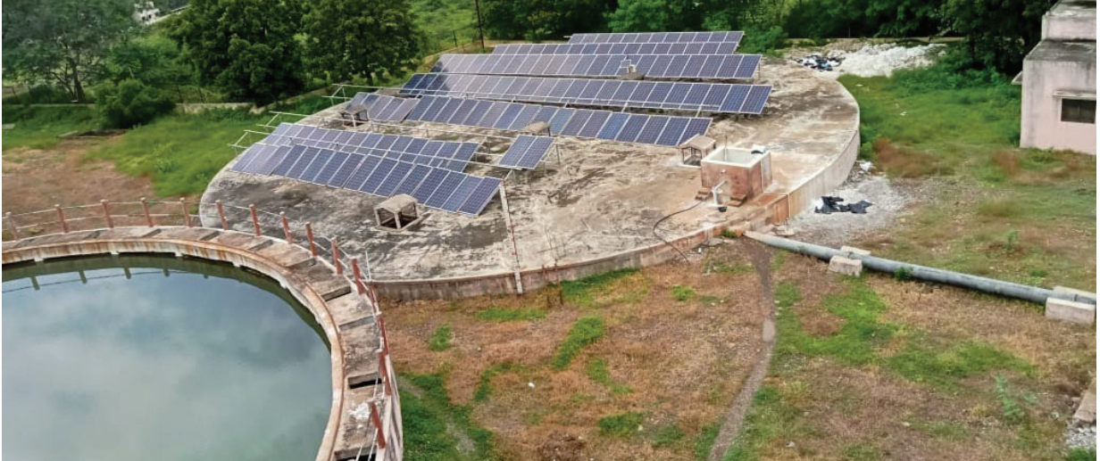
Solarization of Water Treatment Plant
