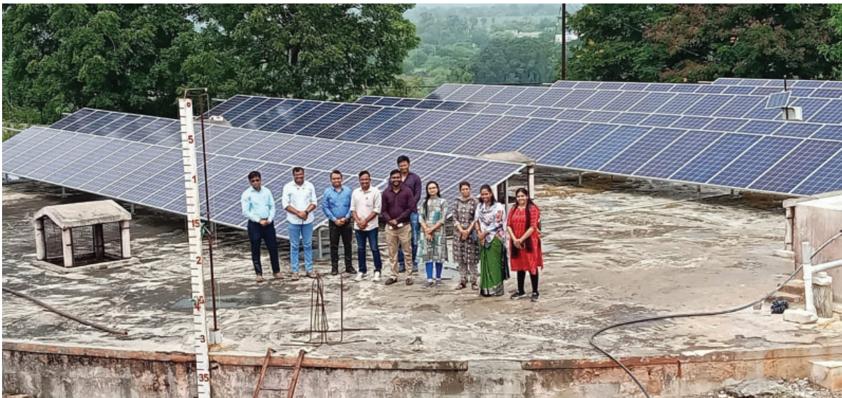
Solarization of Water Treatment Plant (WTP) in Ambarishi Tekdi
